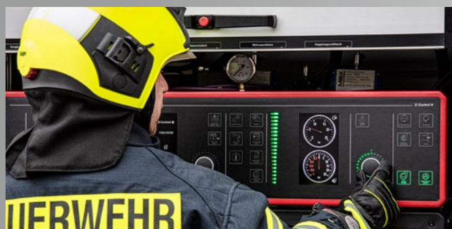
Control and Operation
